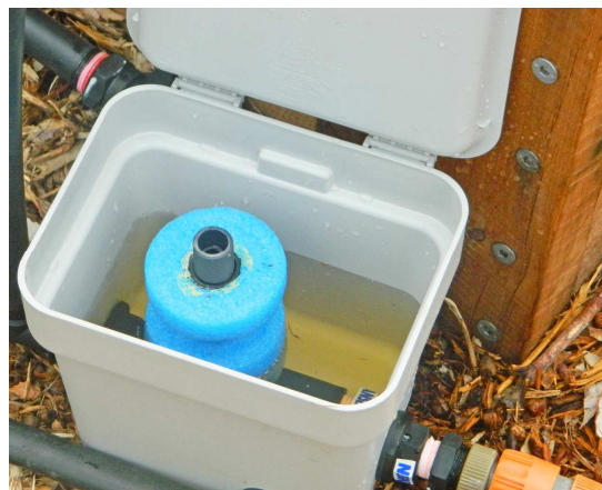
The water level in the controller is the same as the water level in the wicking bed.
