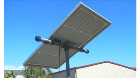
Solar panel mounted on a pole
