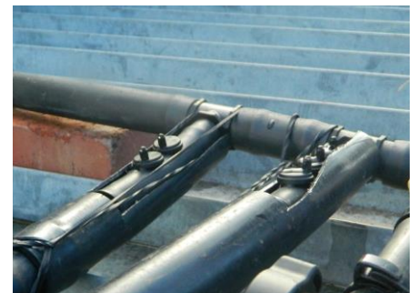
Dripper assemblies for zones 1 & 2 at level 0. The drippers are open to the atmosphere.
