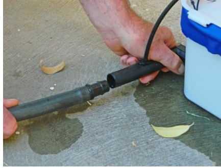
Connect the irrigation application to the controller inlet
