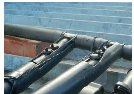
Dripper assemblies for zones 1 & 2 at level 0. The drippers are open to the atmosphere.
