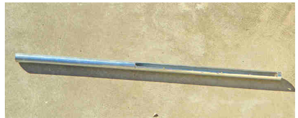
An angle grinder can be used to make a long slot in a length of steel pipe
