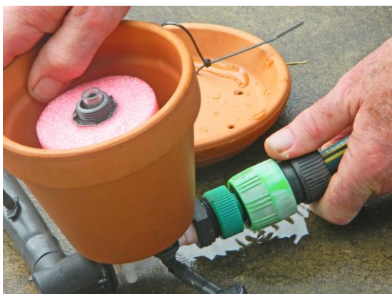
Connect the water supply to the controller inlet
