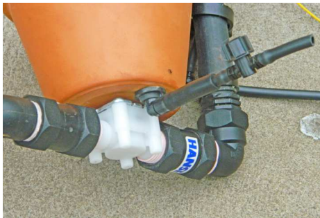
Drain valve and white valve with 15mm inlet and outlet
