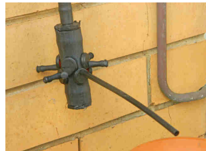
The control dripper drips water into the terracotta saucer and the remaining seven lower drippers should be blocked.
