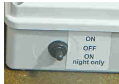
Switch in the ON night time position
