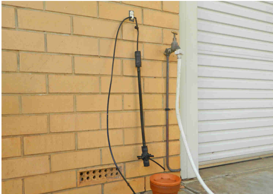
Fractional dripper suspended above the terracotta pot
