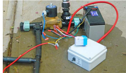
Eleven colour-coded wires connected to the relevant components
